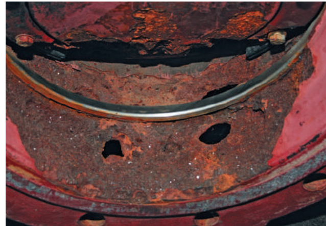
Improper continuous use of butterfly valves as a control valve can result in dramatic material damage, as in this valve opened by 5° after a year in seawater.
